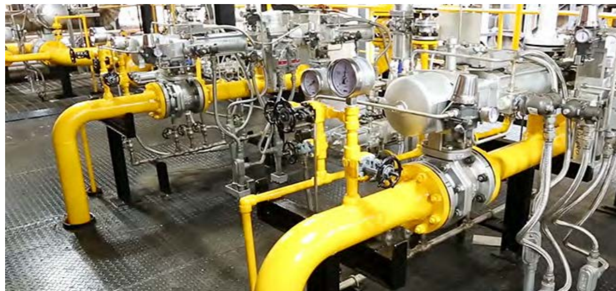
Power boiler only operated by eco-friendly LNG fuel (Ulsan CLX)
